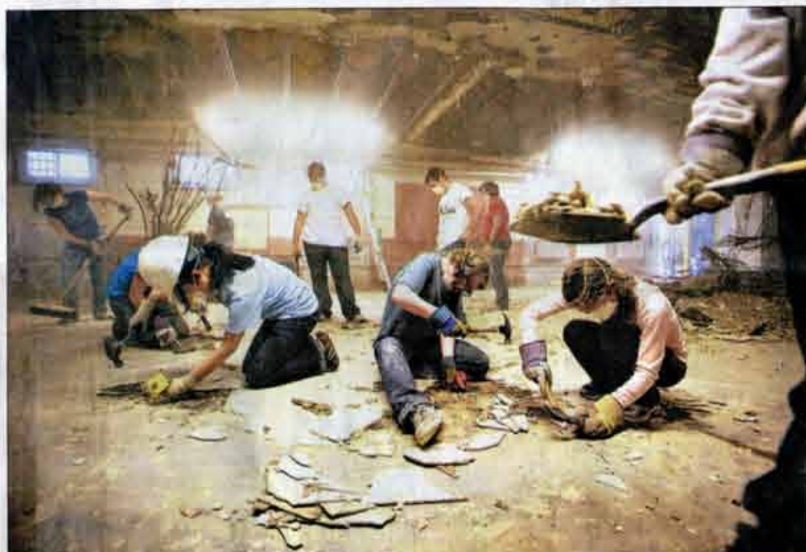
College students pull up and remove tiles in the basement of UrbanPromise's East Side building.
