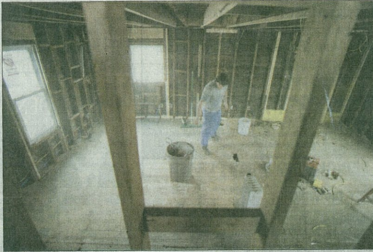
Nick Palladino, a student at Randolph-Macon College in Virginia, helps renovate a building at Urban Promise in Camden.
